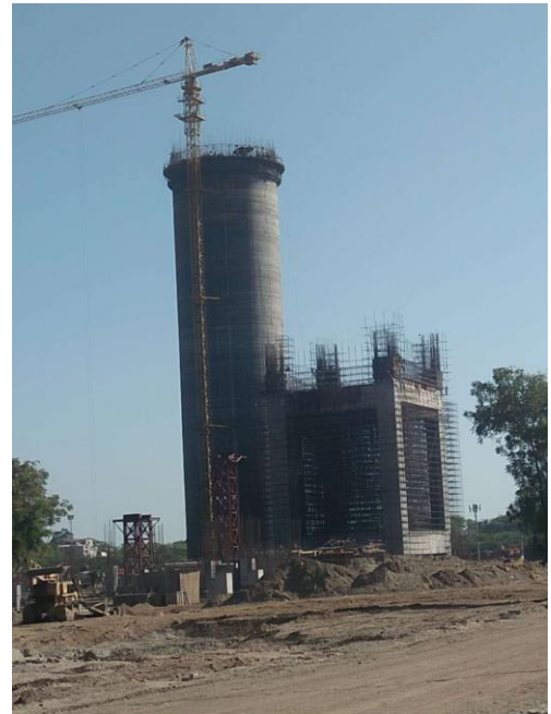
Fig: Cement Silo at Rajashree Cement, Malkhet, Karnataka
