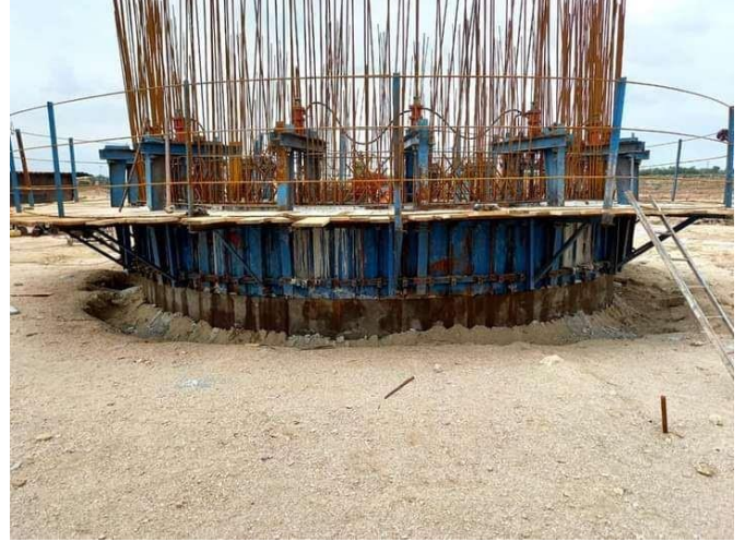
Fig: Reamal Intake Well
