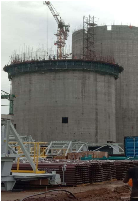
Fig: Clinker and Cement Silo at Satiudyog, Hata, Jamshedpur
